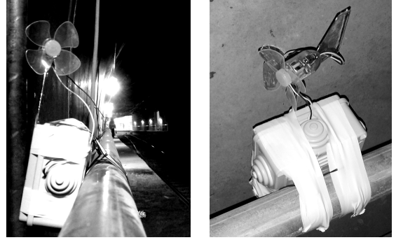
Fig. 5. Snapshot of nodes deployed in a tunnel of the Metro B1 line in Rome.
